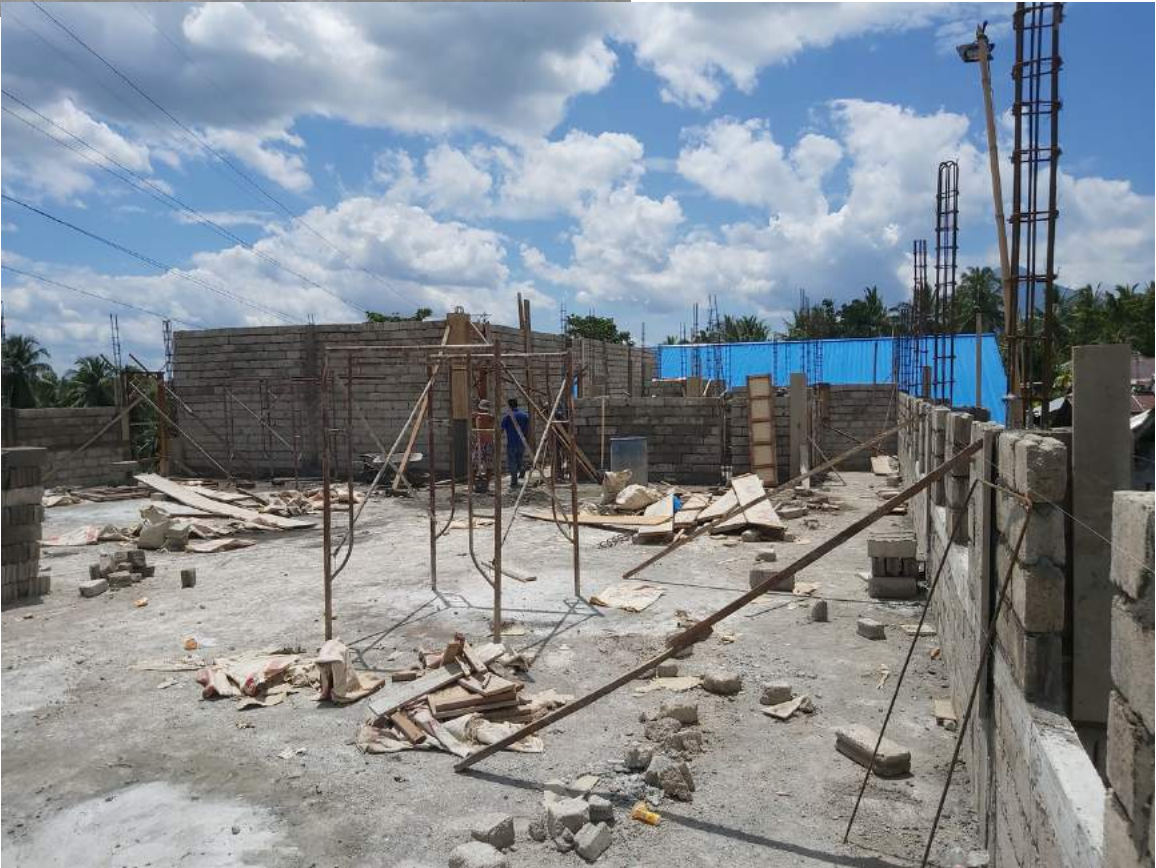
They work fast and have a lot of the walls up on the 2 nd -floor.
